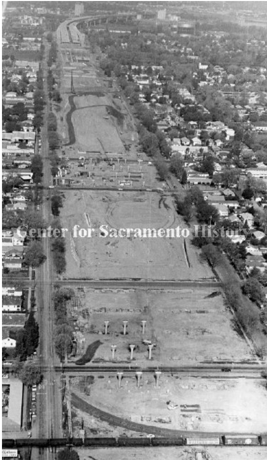
Figure 28: Demolished area of Richmond Grove during freeway construction, view from 19 th Street, 1966 (Center for Sacramento History).
